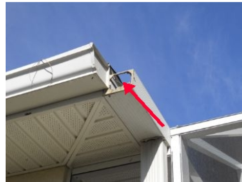
Damage south endcap
