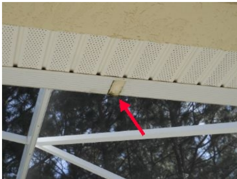
Leaky gutter seam
