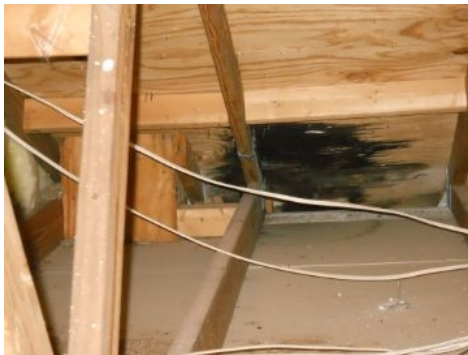
Water staining and wood rot
