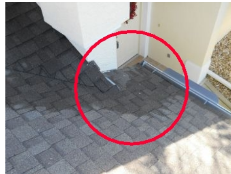
Exterior view of damage area
