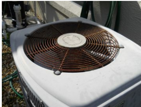
Rust along exterior unit
