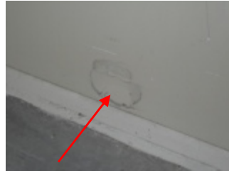
Minor damage along garage wall
