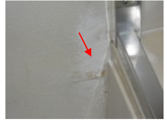
patched area on wall of master bathroom
