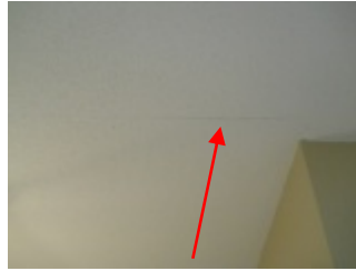
Seam pulling loose along ceiling
