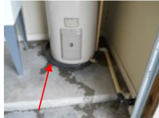
from behind the wall of water heater
